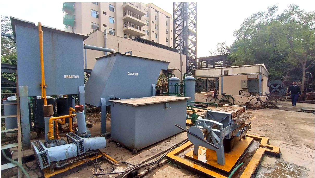
Photograph :- 350 KLD STP & 25 KLD ETP Area
