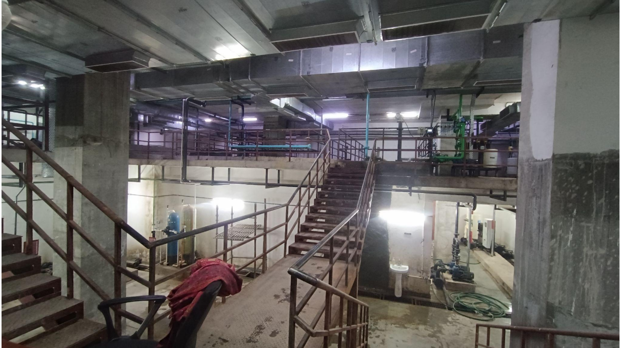
Photograph :- 400 KLD STP & 20 KLD ETP Area
