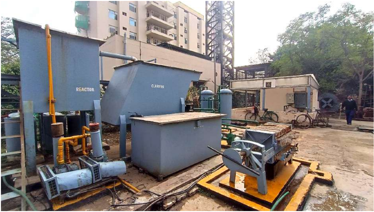
Photograph :- 350 KLD STP & 25 KLD ETP Area
